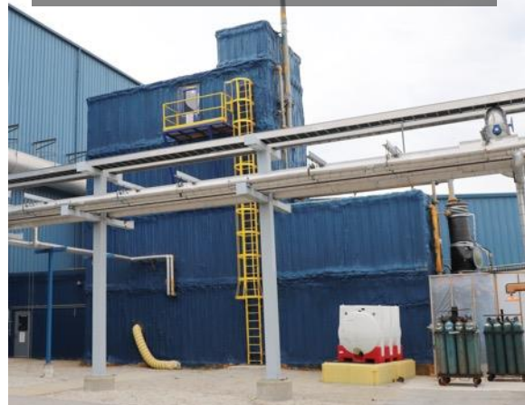
Molten Salt Purification Plant Elmore, OH
