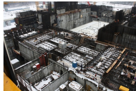
Steam Generator Compartment of Main Building
